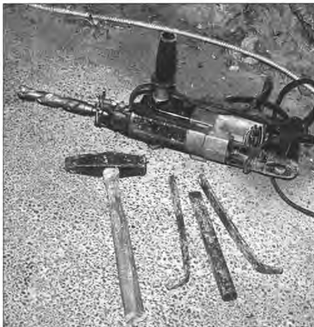
Figure 3. Use a hammer drill with plug and feathers to split large blocks of rock into smaller, safer chunks of rubble. This is a low-impact technique when workers take care to contain the dust that results from drilling.
