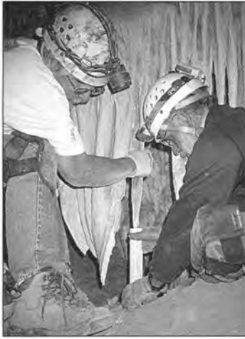
Figure 2. Brace with upward pressure and allow time for the epoxy to cure thoroughly. Steve Wilsey holds the joint in place while Sheridan Stone props the stal with a PVC pipe.
