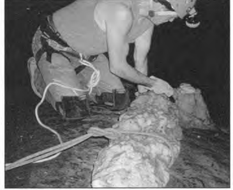
Figure 2. Since the repair is performed on a sloping flowstone surface, cavers and large broken pieces are secured with safety lines.
