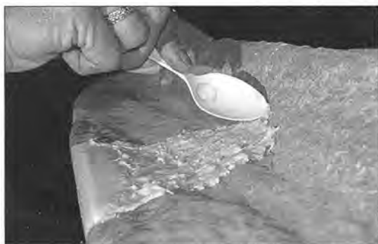
Figure 4. After allowing the epoxy to set up for several hours, we used a plastic spoon to create a base texture in the thickened epoxy mixture.
