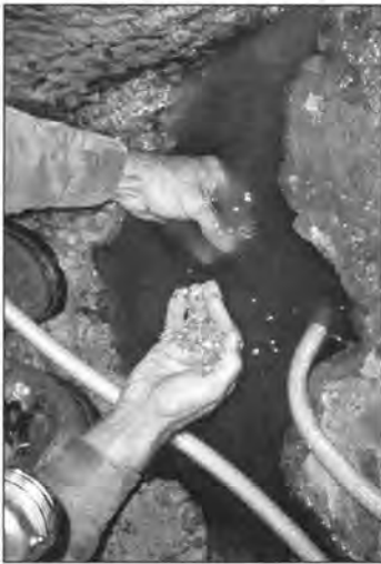
Figure 3. Thoroughly clean the repair area. Remove mud and debris before attempting to reconstruct rimstone dams with cement products.
