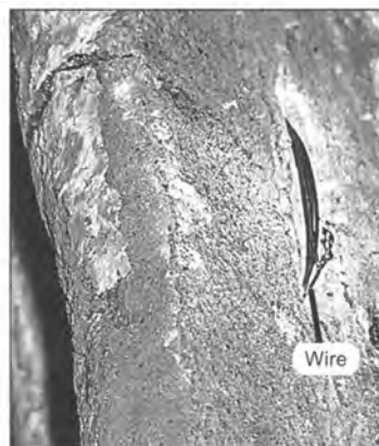
Figure 7. To reinforce the pin and epoxy repair, stainless steel wire is threaded through small drill holes above and below the upper break joint. Alongside the wire, there are additional stainless pins installed at an angle up through the break joint and into the ceiling.
