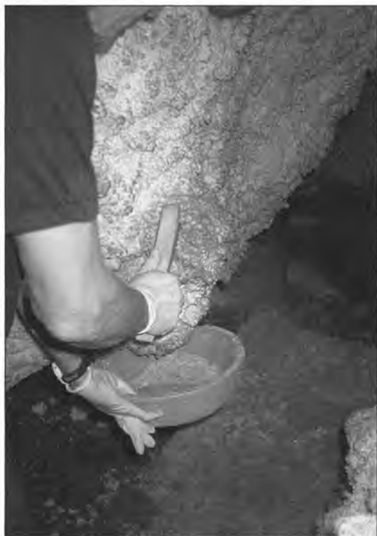
Figure 2. A tile grout brush or a brush with stainless bristles will clean gypsum surfaces. Catch all the scrapings and stray bristles. Always use gentle strokes.
