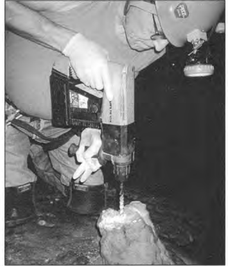
Figure 4. Jim Werker drills a larger hole in the stump to receive the stainless steel pin.
