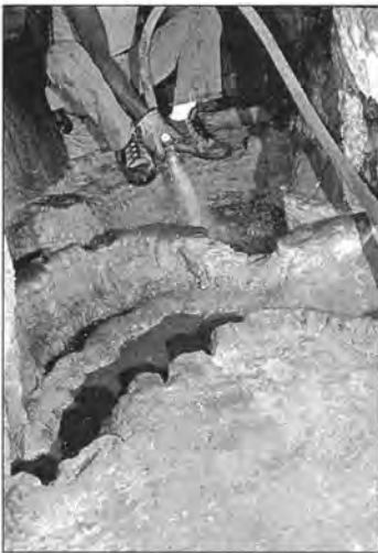
Figure 6a. These three photos show the progression of rimstone repair in Happy Jack Cave, Arizona. First, clean the repair site. All surfaces should be as wet as possible before applying patching materials.
