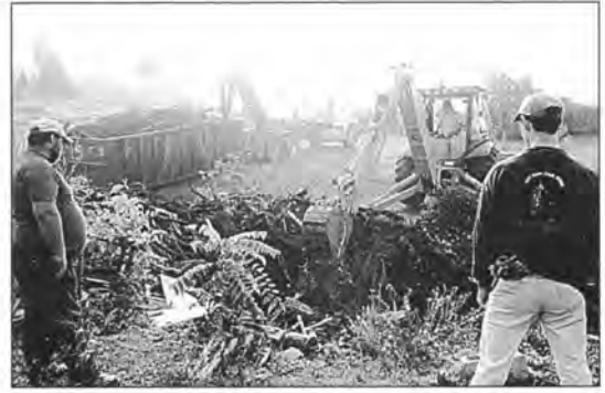
Figure 2. County workers and caver volunteers watch the heavy-equipment operator performing cleanout work as part of a joint venture between the Virginia Department of Conservation and Recreation, the Cave Conservancy of the Virginias, and the VPI Cave Club Student Grotto of the NSS.
