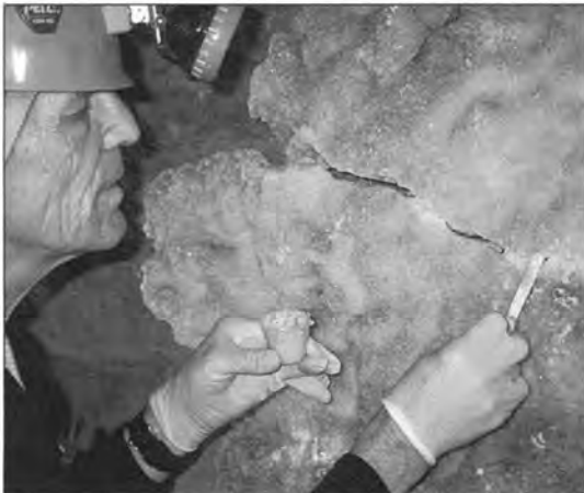
Figure 4. Jim Werker fills seams and gaps with a thick mixture of epoxy and gypsum dust.
