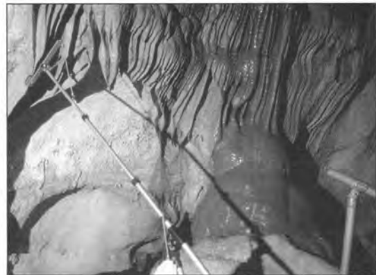
Figure 7. Use a similar technique for stalactite repairs in inaccessible locations.
