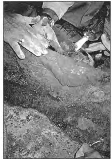
Figure 5. Use trowels, brushes, wires, and sculpting tools to shape the cement and match the texture of reconstructed sections to the original. Wear disposable vinyl gloves to help protect cavers' hands.
