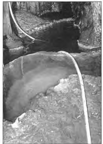
Figure 6c. This view shows the completed rimstone dam. Repaired rimstone dams should retain water like the originals.
