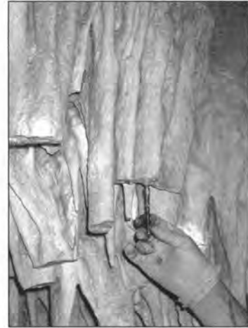
Figure 7. Stainless steel all-thread is epoxied into the drill hole to provide stabilization for the stalactite repair.
