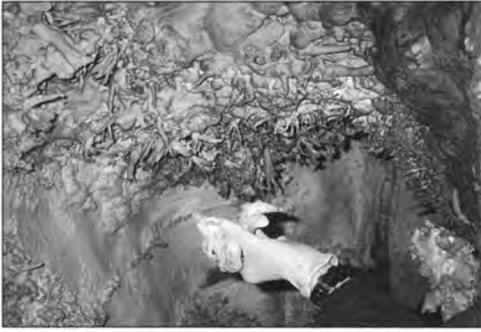
Figure 1. The empty scar where this speleothem was broken off is apparent on the helictite-covered wall. See the repair in Figure 2.
