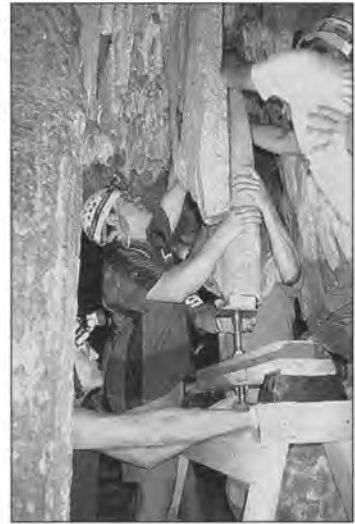
Figure 5. Dennis Hoburg and others position the large stalactite while Jim Werker adjusts the screw jack support structure.
