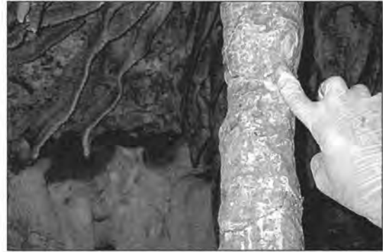
Figure 7. Press the epoxy and rock dust mixture into cracks and holes. Create texture as the epoxy is curing.
