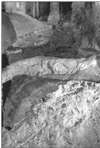
Figure 6b. Next, use gloved hands and various tools to sculpt cement and fill in missing sections of the rimstone dams.
