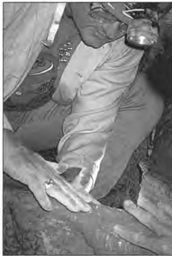
Figure 4. Jerry Trout uses quick-setting cement to manually sculpt missing pieces of rimstone.
